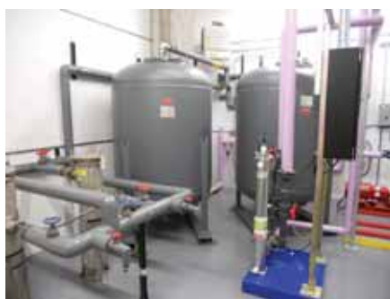
Top: Gateway Village earned LEED Gold with the help of its groundwater reclamation system. Bottom: The treatment system is carefully designed to maintain the same heat transfer efficiency as with potable water.
